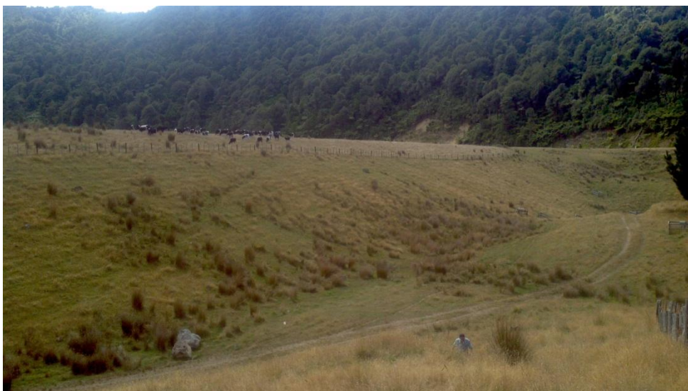
Photo 1: View of Saddle Embankment from Trig J. Note seepage and erosion areas defined by reed grass
