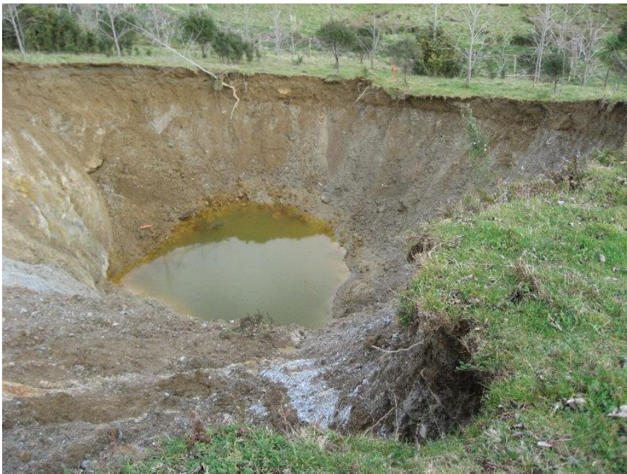
Photograph 1: View of sink hole on 26 July 2013 from the upslope (east) side
