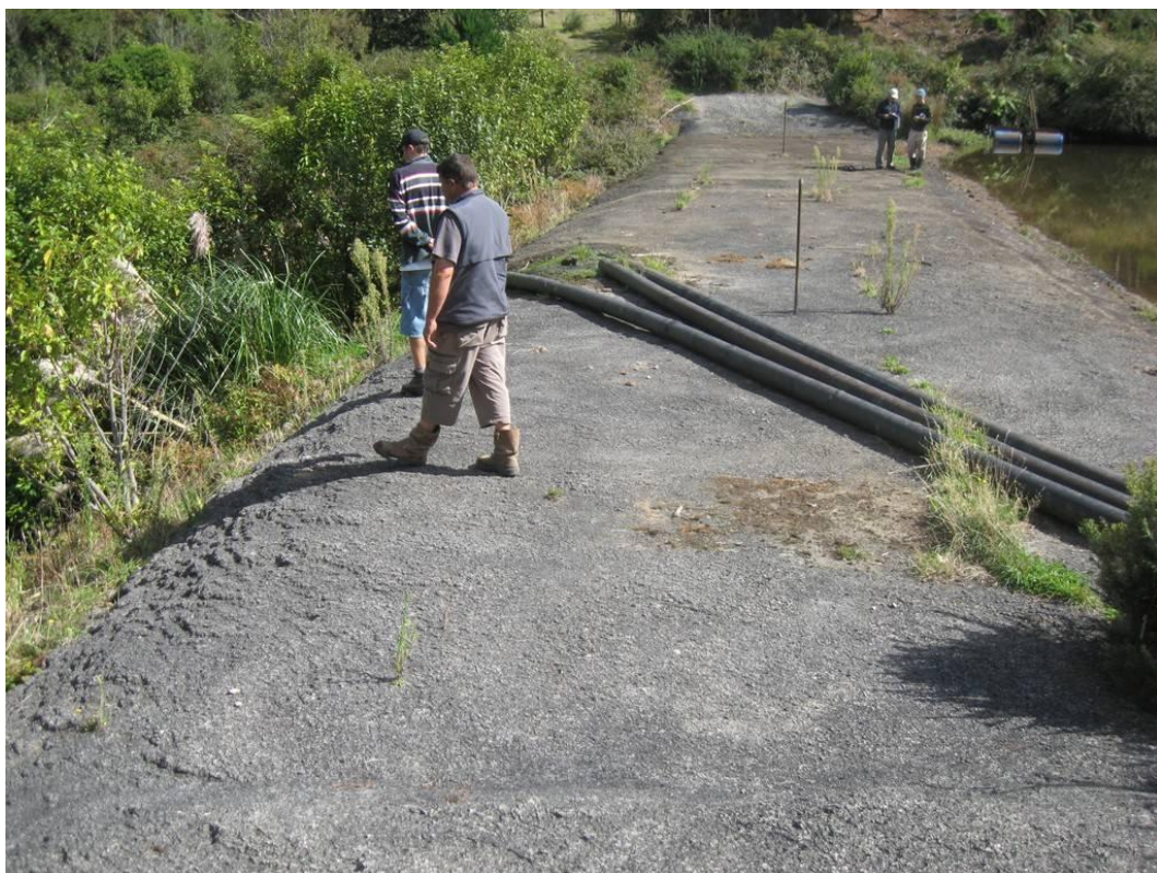
Photograph 8. SYSD crest/spillway looking from left abutment, with low point in crest at the far end
